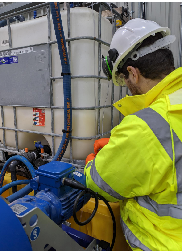
Ionic Technologies' Belfast demonstration plant
